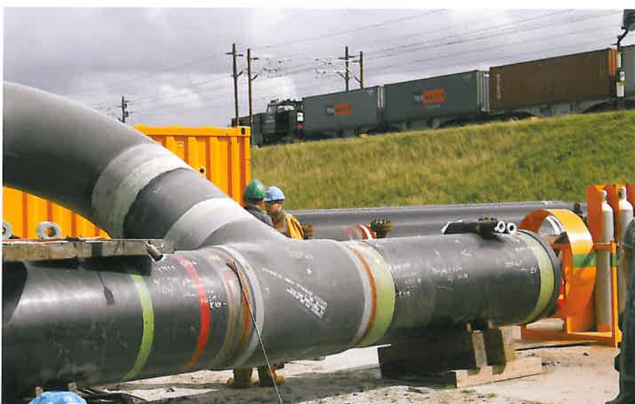
The tie-in pipe being assembled above ground. The field joints for the tee are protected with the STOPAQ system.
