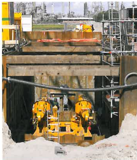
The launch pit for the Hartelkanaal crossing. The pit is being prepared to accept the pipe sealing unit and the tunnelling machine. Visible also is the two-piston pipe-thrusting unit onto which the clamping unit will be fixed, be used to push the pipe into the microtunnel.
